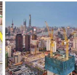
Construction Site: "Keep Out"
